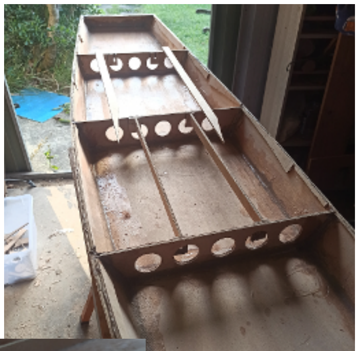
Above: Deck stringers layed out. Also note the rough cut inwales out of offcut materials
